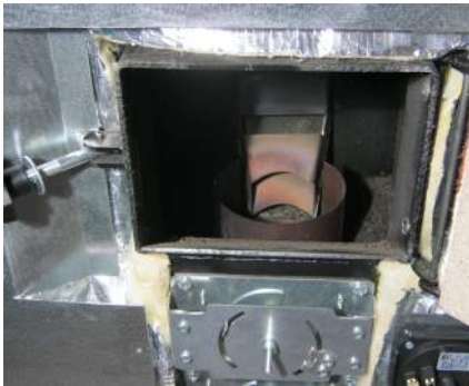
Boiler with integrated burner
