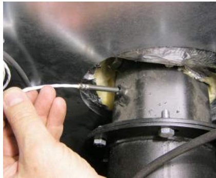
Flue gas temperature sensor
